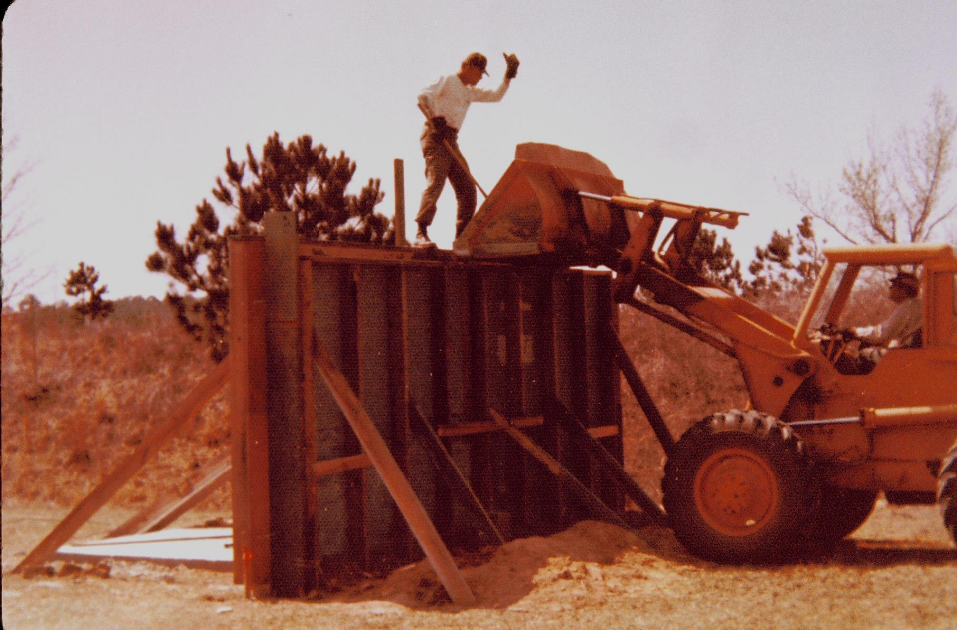
We built the forms from scrap plywood and 2x6s and poured the cement into the open top of the forms. Sgt. Moeller is directing the front end loader with the cement. As a side note, we didn't reinforce the bottom half of the form well enough and it bulged requiring extra cement.
